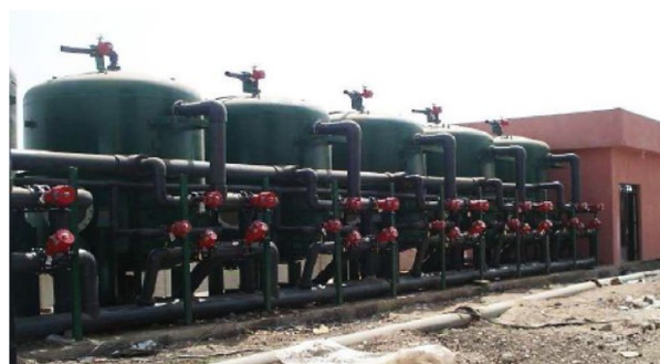
Figure 9. Rapid sand filters following the Oxidizer at Bani Murr WTP to filter out the oxidized iron and manganese.
