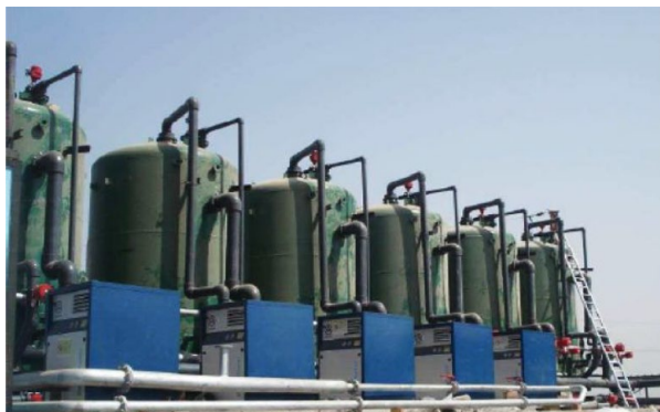
Figure 8. Oxidizers at Bani Murr WTP.
