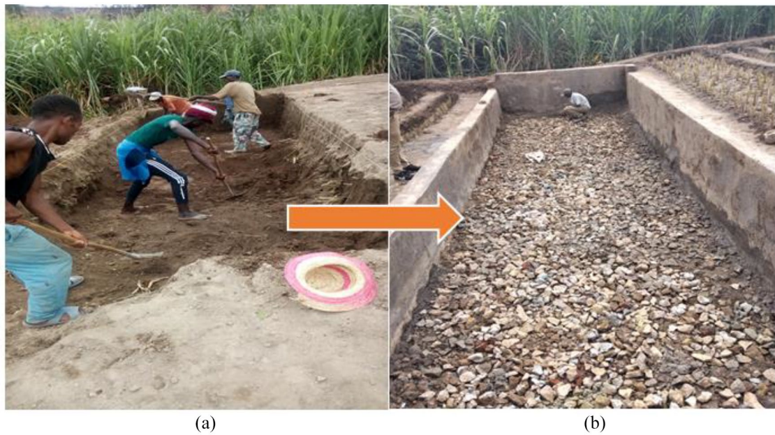
Figure 6. Construction of open space between 2 wetlands: (a) during excavation and (b) after construction.
