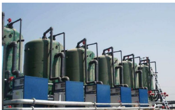
Figure 8. Oxidizers at Bani Murr WTP.
