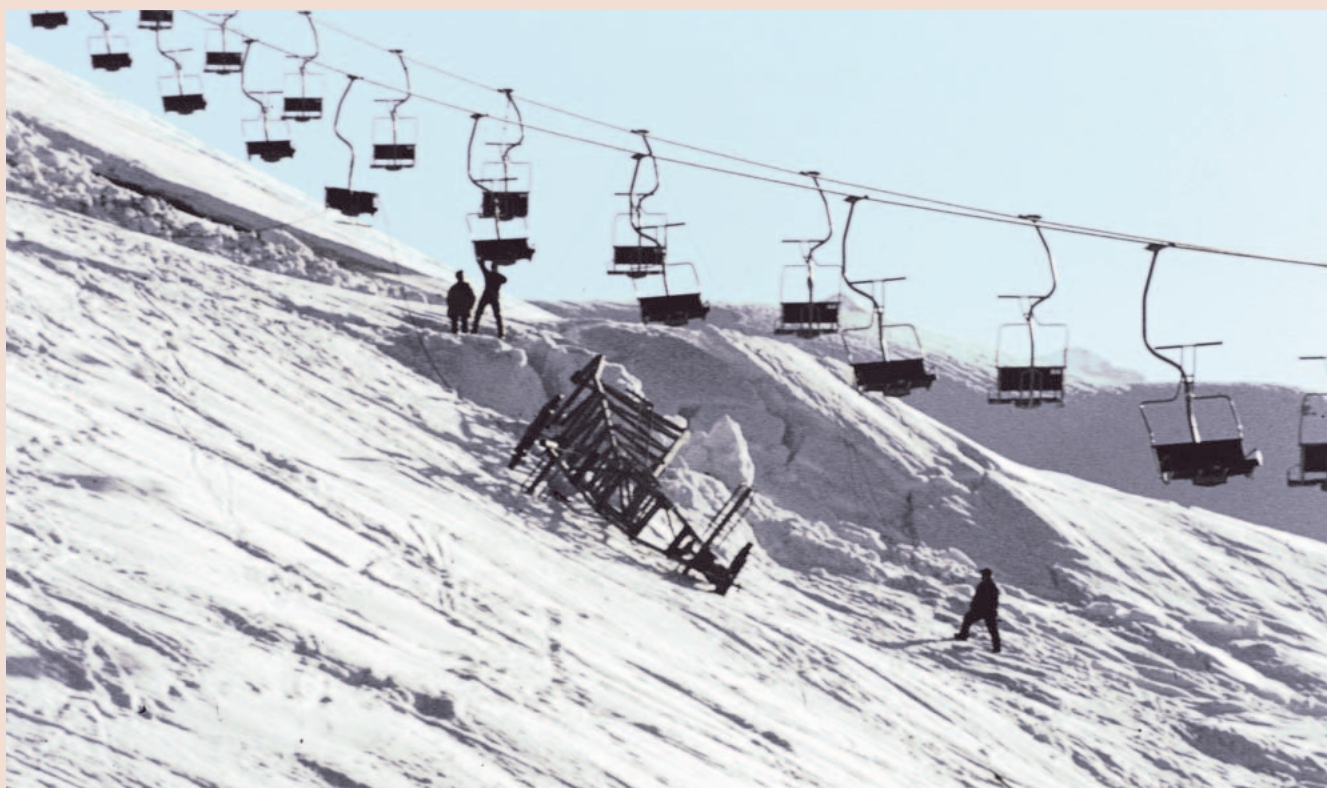
FIGURE 3 Chair lift pylon damaged by snow pressure on 14 March 1999, in Hasliberg (Canton of Berne, Switzerland). (Photo courtesy of SLF)
