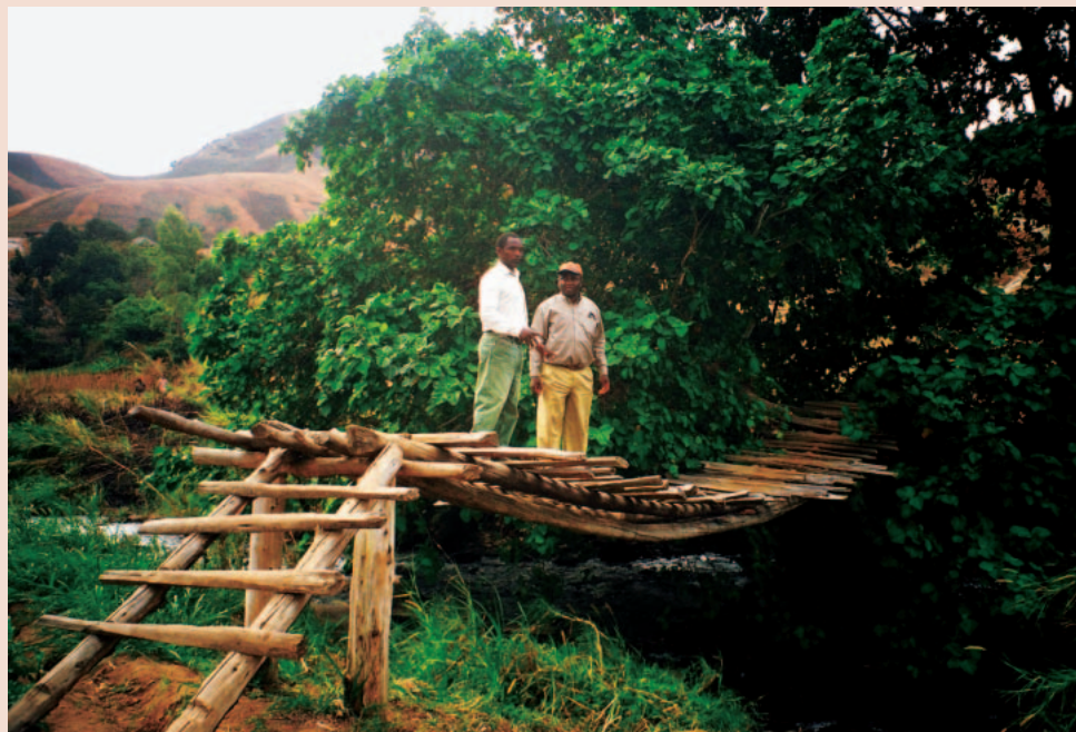
FIGURE 3 The Lubigwa pedestrian bridge, built using traditional methods pre-dating the new suspension technology. (Photo by Mr. Kanyunyu, ITECO)
