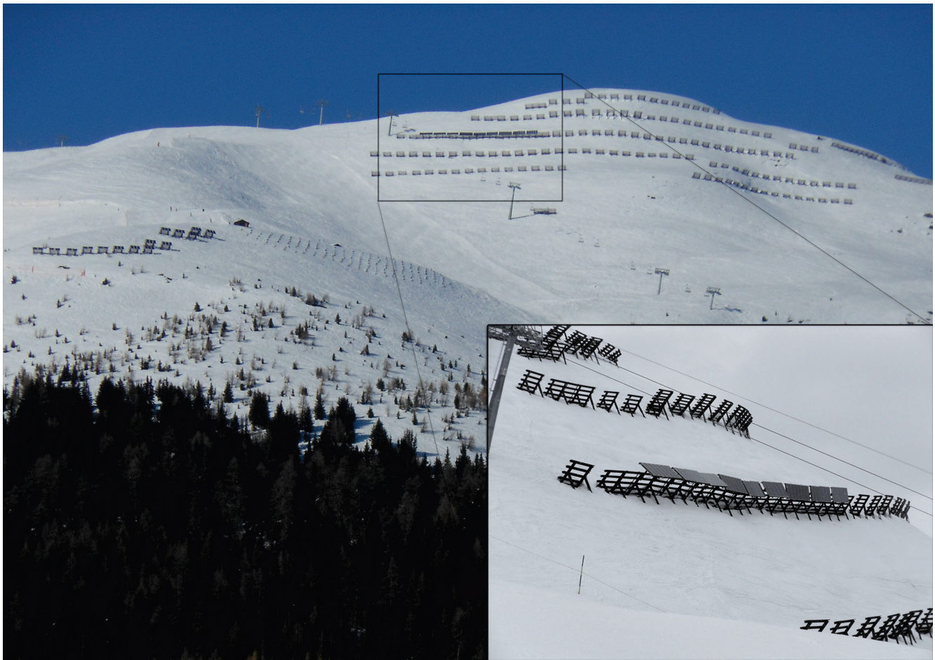
FIGURE 1 Avalanche barriers with photovoltaic installations in the ski area near Bellwald. On the left side, the panels are installed individually; on the right side, also shown in the inset, the panels are connected. (Photos by Annina Michel)
