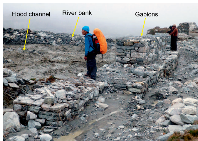
FIGURE 3 Gabions constructed near Chukhung village in 2016, following a threatening englacial flood from the Lhotse glacier in 2015. Local lodge owners credited the gabions with protecting the village during a second flood in 2016. (Photo by Alton C. Byers)
