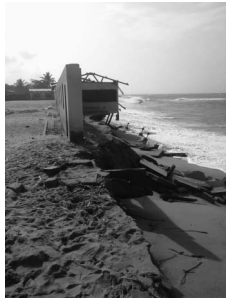
Figure 4. Collapsed school building in Fuvemeh community, which illustrates the effect of coastal erosion on vulnerable delta communities (taken June 2016).
