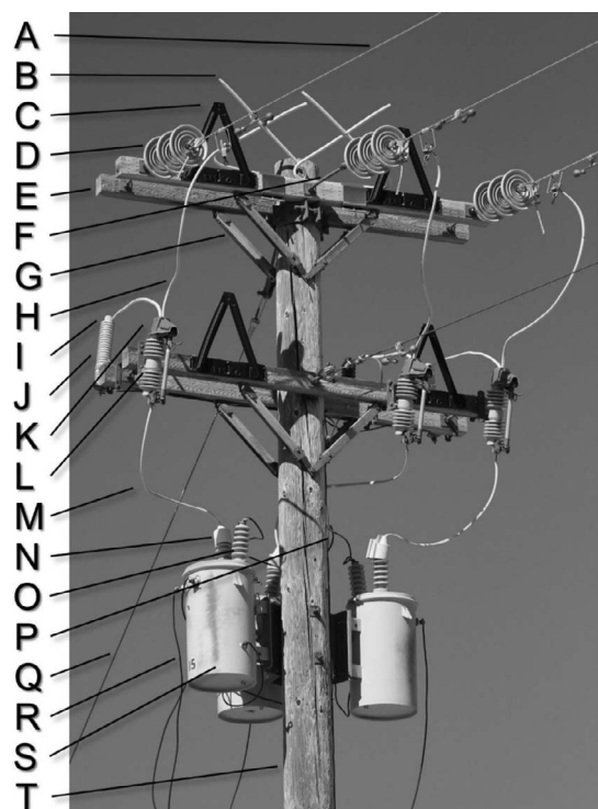
Figure 2. Common power pole (pole) components useful in understanding retrofitting mistakes for birds electrocuted between January 2013 and December 2015 on poles described as retrofitted, in Arizona, Colorado, Idaho, New Mexico, Utah, and Wyoming, U.S.A. See APLIC (2006), Dwyer et al. (2013), and APLIC (2015) for additional illustrations. See Table 1 for component names.
